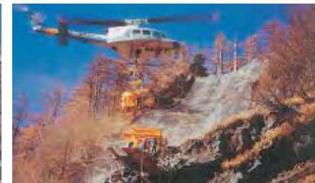
●富士山大沢崩れ源頭部対策 Landslide Prevention in Osawa Area on Mt Fuji 標高2,200mより上流の大沢崩れ源頭域は、もっとも崩壊の激しい区域であり、土石流の発生源です。高標高である大沢崩れから流出する土砂量を軽減する土木工事は、施工技术・資材運搬手段などの技術的な課題や環境・景観問題などがたくさんあります。このため昭和55年より調査工事が開始され、現在までに17種類の試験施工を行っています。 Osawa area located at an elevation of 2200m is frequently damaged by severe landslides. A landslide originated in the area often turns into a debris flow. Civil engineering works for decreasing the amount of sediment flowing down from Osawa area pose a number of problems including technical issues like construction techniques and means for transporting materials, environment, landscape and other numeric problems. To attack these problems, pilot works have been under way since 1980. So far seventeen types of pilot works have been performed.
