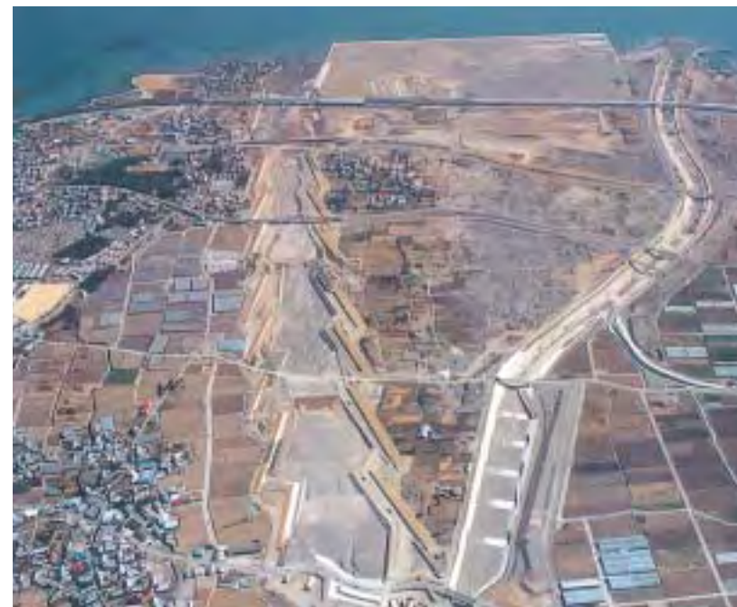
導流堤と遊砂地 Training dikes and sand pockets
