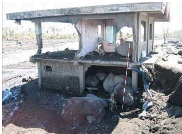
Photo.7 Damage at Daraga Town(2)
