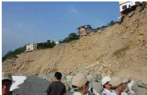
Photo-1: Tremendous bank erosion
